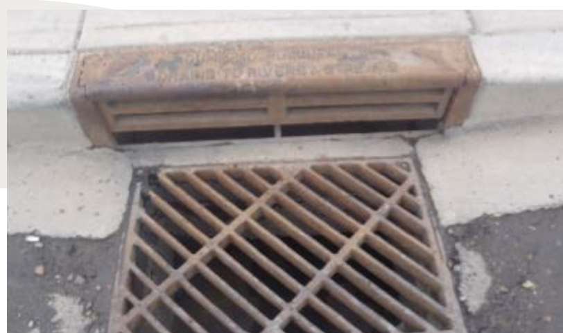
Photo 2 Dump no pollutants, drains to river
